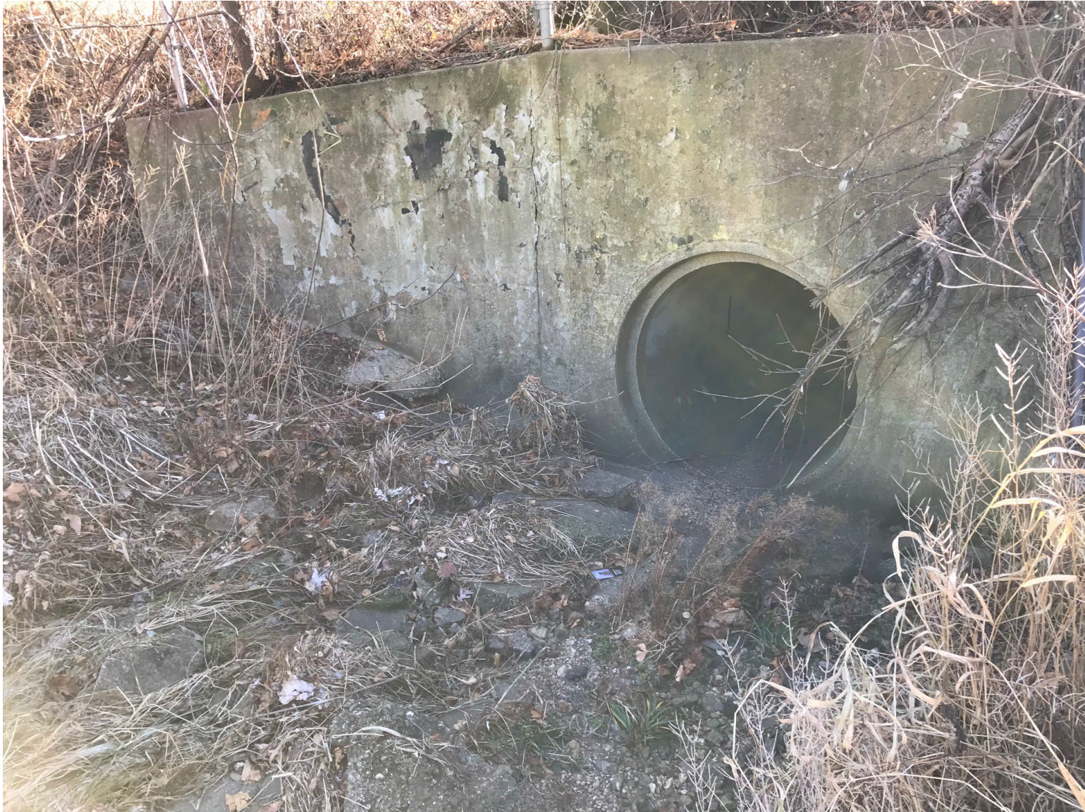
Raymond Road 48" RCP with vertical headwall and socket end (0.2 entrance loss coefficient)
